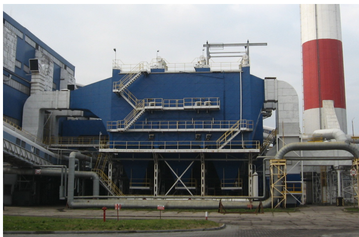
Fig. 1. Electrostatic precipitator in Thermal-Power Station.
